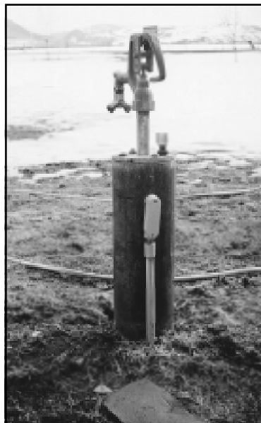
Figure 5.3.6 Poor hydrant installation
