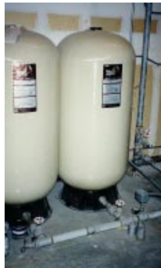
Figure 5.7 Captive air tanks
